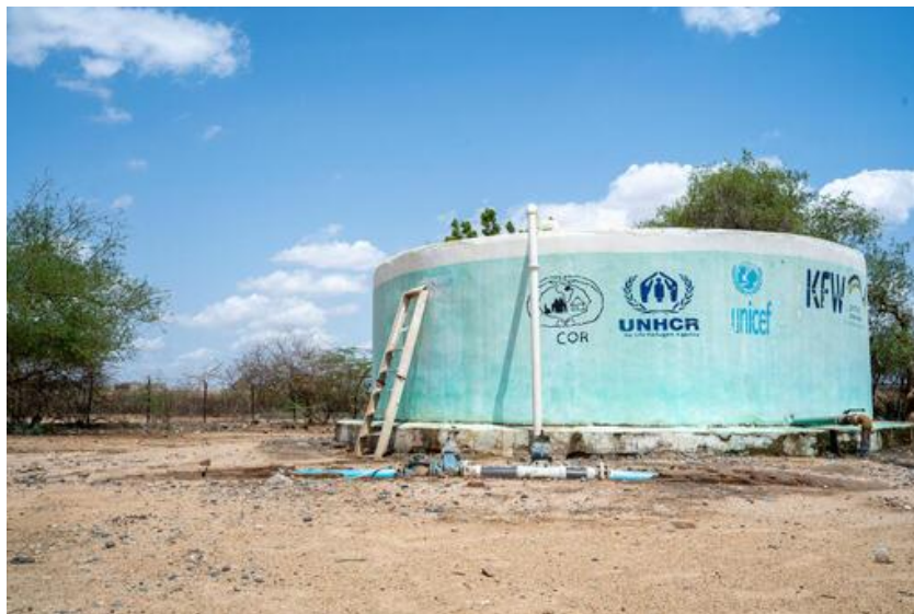
Storage tanks at the water station in Wadsharefey refugee camp in Kassala state. ©UNICEF/UNI851843/Saif
